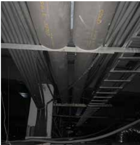
PE temperature regulation replaced by office and hallway chilled water piping
