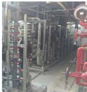
Acid/alkaline waste water recycling system
