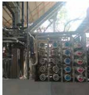
EPI waste water recycling system
